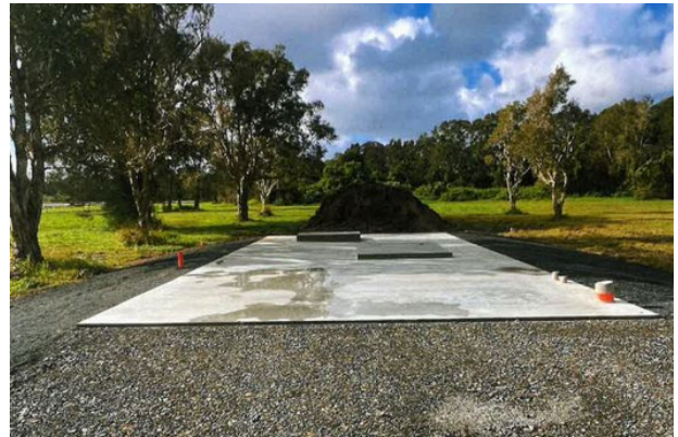
Ballina new irrigation system pump station
